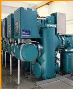
Gas-Insulated Switchgear GIS
