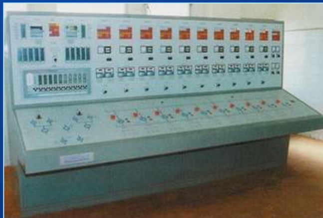
BALOZA Pumping station control desk
