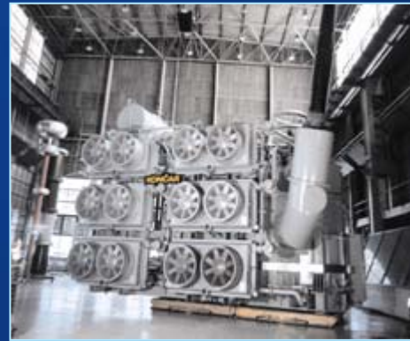
TPP FARAKKA 1f, 420 kV/ 200 MVA INDIA
