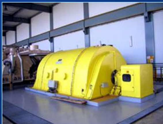
CCPP ZAGREB 1 (OF 3) 80 MVA CROATIA
