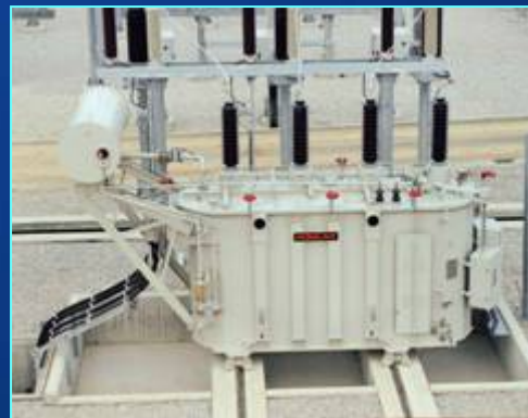
SS ŽERJAVINEC 20 MVA 110±10x1,5%/21(10,5)/10,5kV CROATIA
