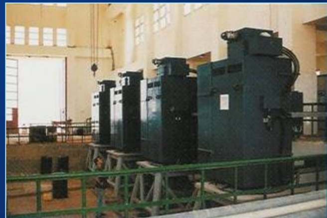
KILO 12,5 1400 kW Pump drive motors
