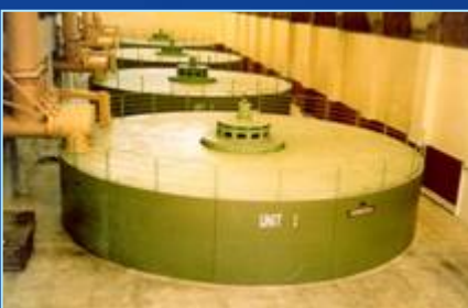
HPP SHIRORO, 4 x 176,5 MVA NIGERIA
