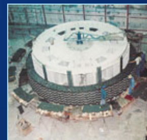
HPP HADITHA, 6 x 128 MVA IRAQ
