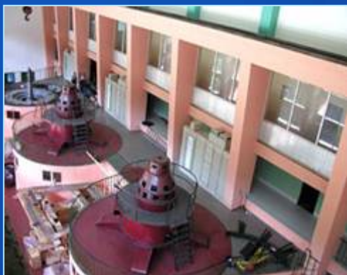
HPP GOJAK, 3 x 20 MVA CROATIA
