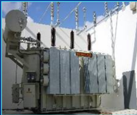
SS REKOLA 40 MVA 115±9x1,67%/21 kV FINLAND
