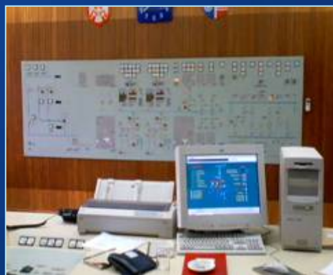
HPP BOČAC, 2 x 65 MVA BOSNIA AND HERZEGOVINA
