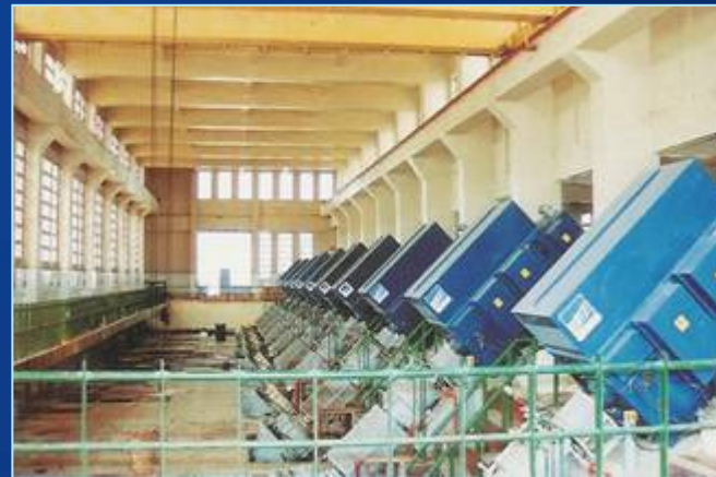
EL SALAM No.4 Main pump drive motors
