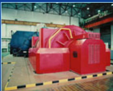
TPP PLOMIN 2, 1 x 247 MVA CROATIA
